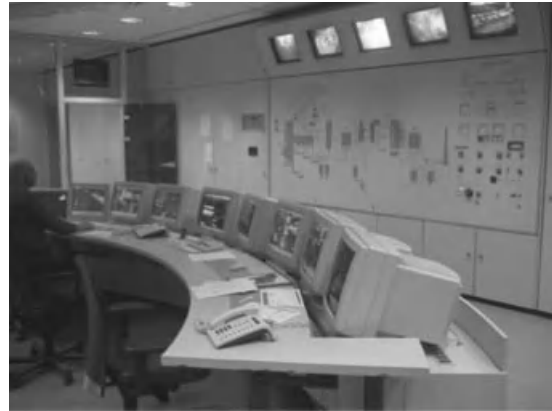
Figure 15 Depiction of a typical process control workstation. (Courtesy of BKB Göppingen.)
