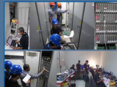
• Power Plant Control System
