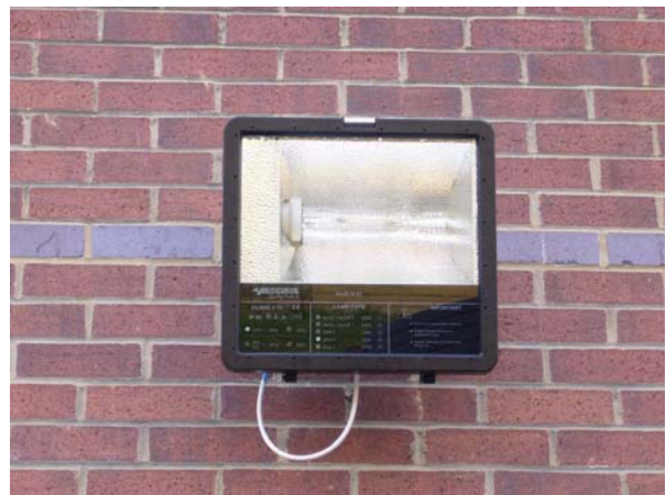
Figure 8.9 Typical security lighting
