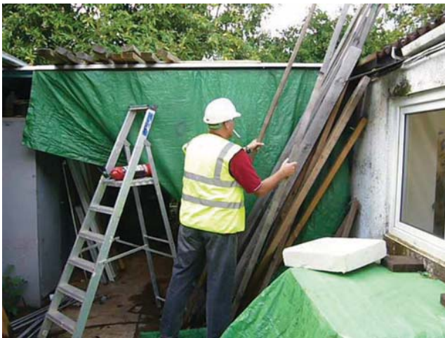
Figure 5.9 Building contractors have the potential to increase fire risk
