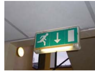
Figure 9.53 Maintained emergency exit box
