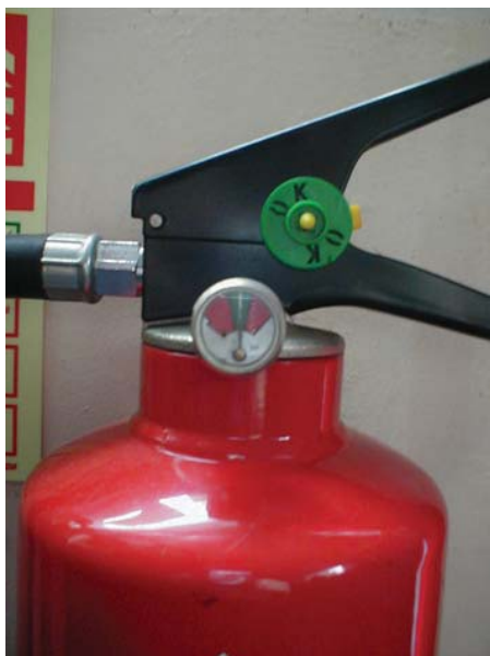
Figure 9.68 Pressure gauge on the neck of a water extinguisher
