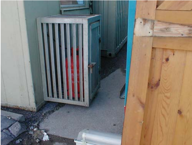
Figure 8.20 LPG cylinder storage facility
