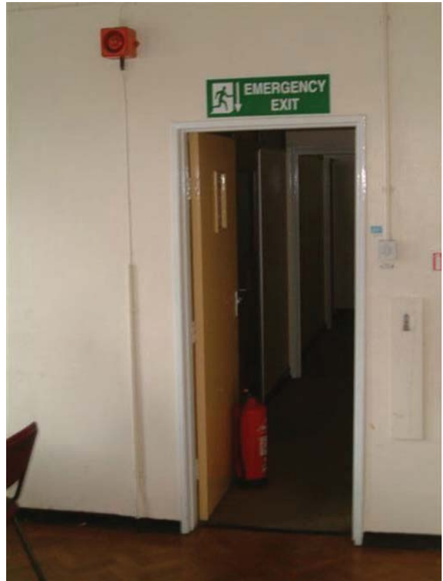
Figure 4.16 Routine violations of basic safety systems indicate a poor safety culture – wedged fire door
