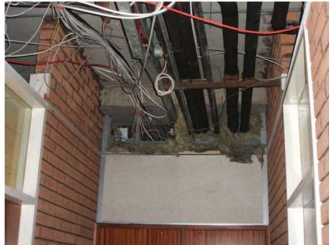
Figure 11.10 Building works which have resulted in the breaching of a fire compartment wall
