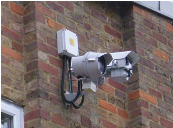
Figure 8.10 CCTV with infrared lights reduce the likelihood of arson attack
