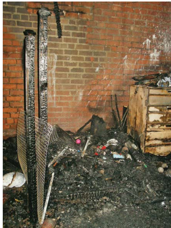
Figure 12.8 The result of an arson attack on an external shed
