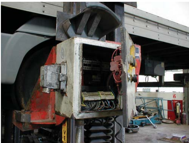
Figure 12.3 Unguarded electrical machinery which has the potential to cause injury in many ways including starting a fire
