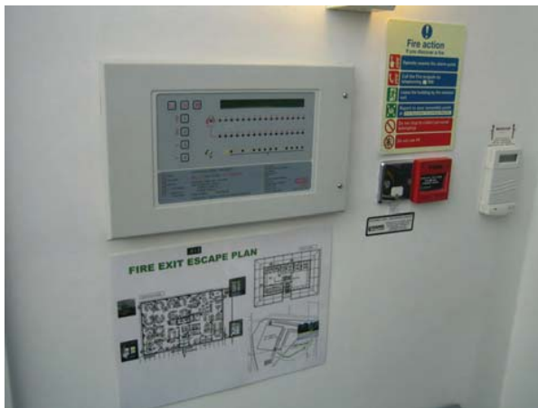
Figure 9.79 Typical fire alarm panel
