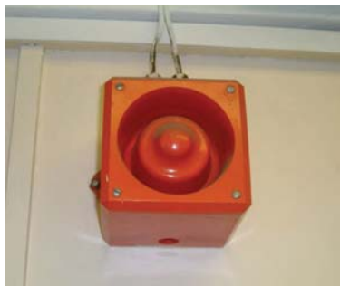
Figure 9.81 Audible fire alarm
