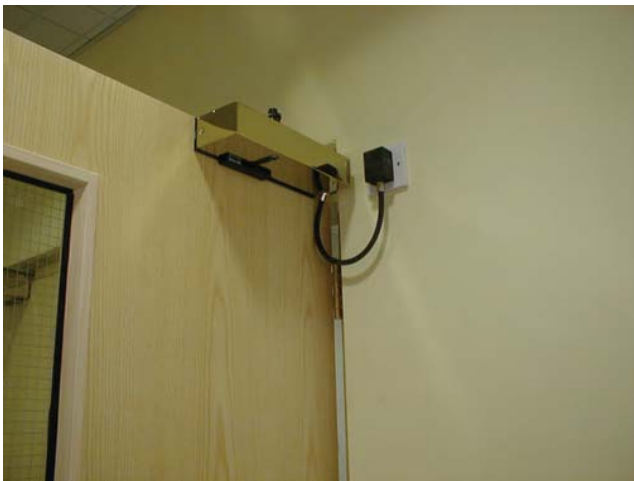
Figure 5.13 A fire door retaining device – an example of the application of technical progress
