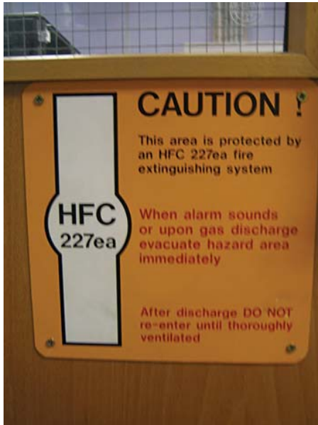
Figure 9.66 Typical warning sign to a computer room fitted with a flood system
