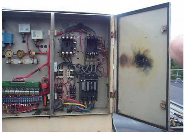
Figure 12.20 Damage to electrical distribution cupboard
