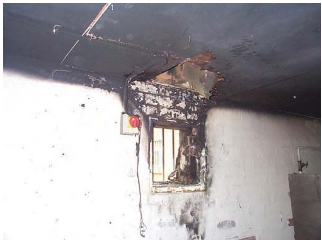
Figure 12.19 Damage to Vent Axia
