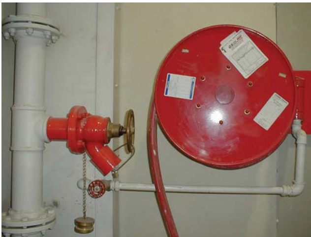
Figure 3.3 Fire fighting equipment must be appropriate and adequately maintained
