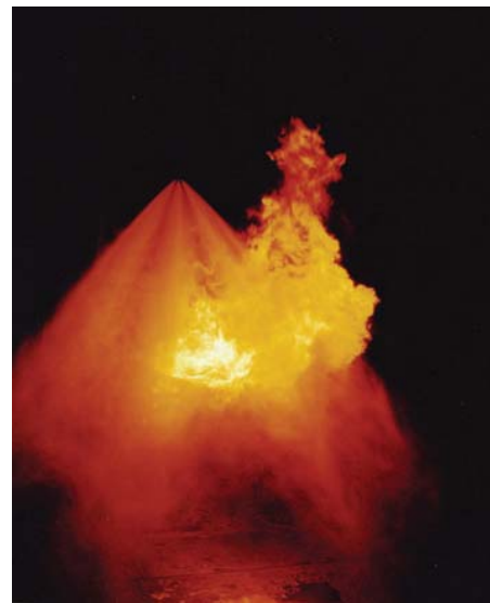
Figure 9.67 High pressure water mist system in operation
