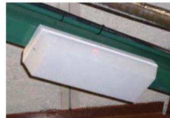
Figure 9.55 Non-maintained satellite emergency light
