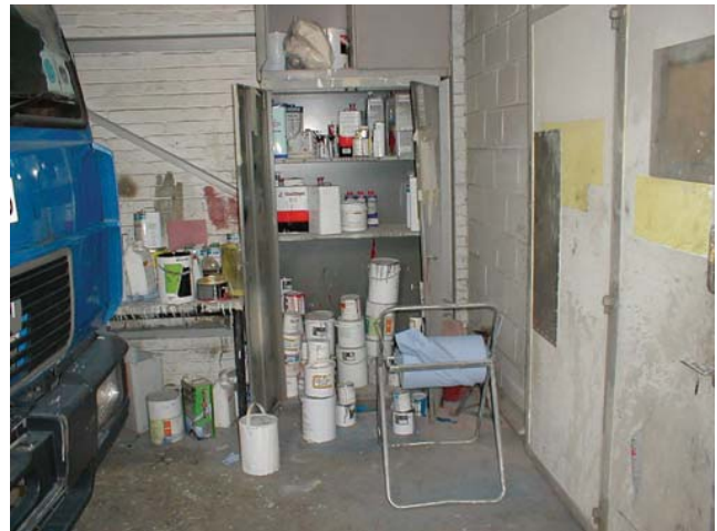
Figure 8.5 Poor storage arrangements for flammable materials
