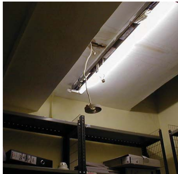
Figure 12.12 The result of contractors working on the fire alarm system – removal of detector head
