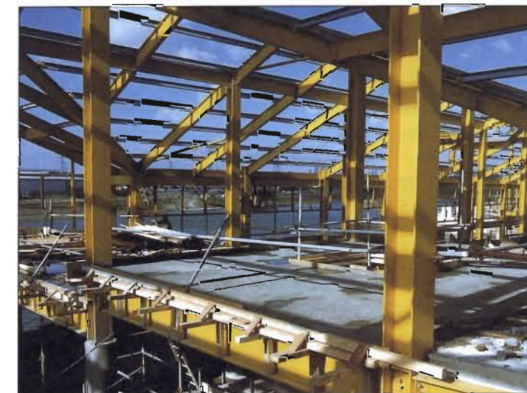
Figure 3.4 Steelwork of various sizes in a framed building. Part concrete "plank" and part poured concrete floor. Note concrete cladding on lower column. Photo: Essex Fire Brigade.
