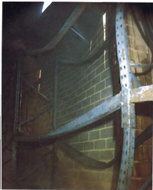
Figure 6.1 Blockwork wall severely distorted but still intact following a fire. Photo: Cheshire Fire Brigade.
