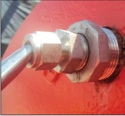
Figure 7.4. Improperly Installed Tubing
