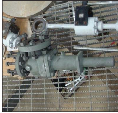
Figure 7.5. Improper Handling of Pressure Safety Valve
