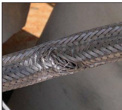
Figure 7.3. Damaged Instrument Cable
