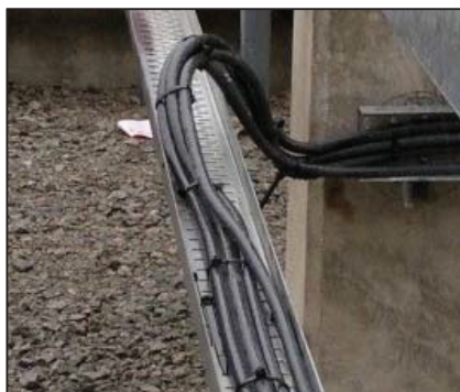
Figure 7.2. Improperly Installed Electrical Cables
