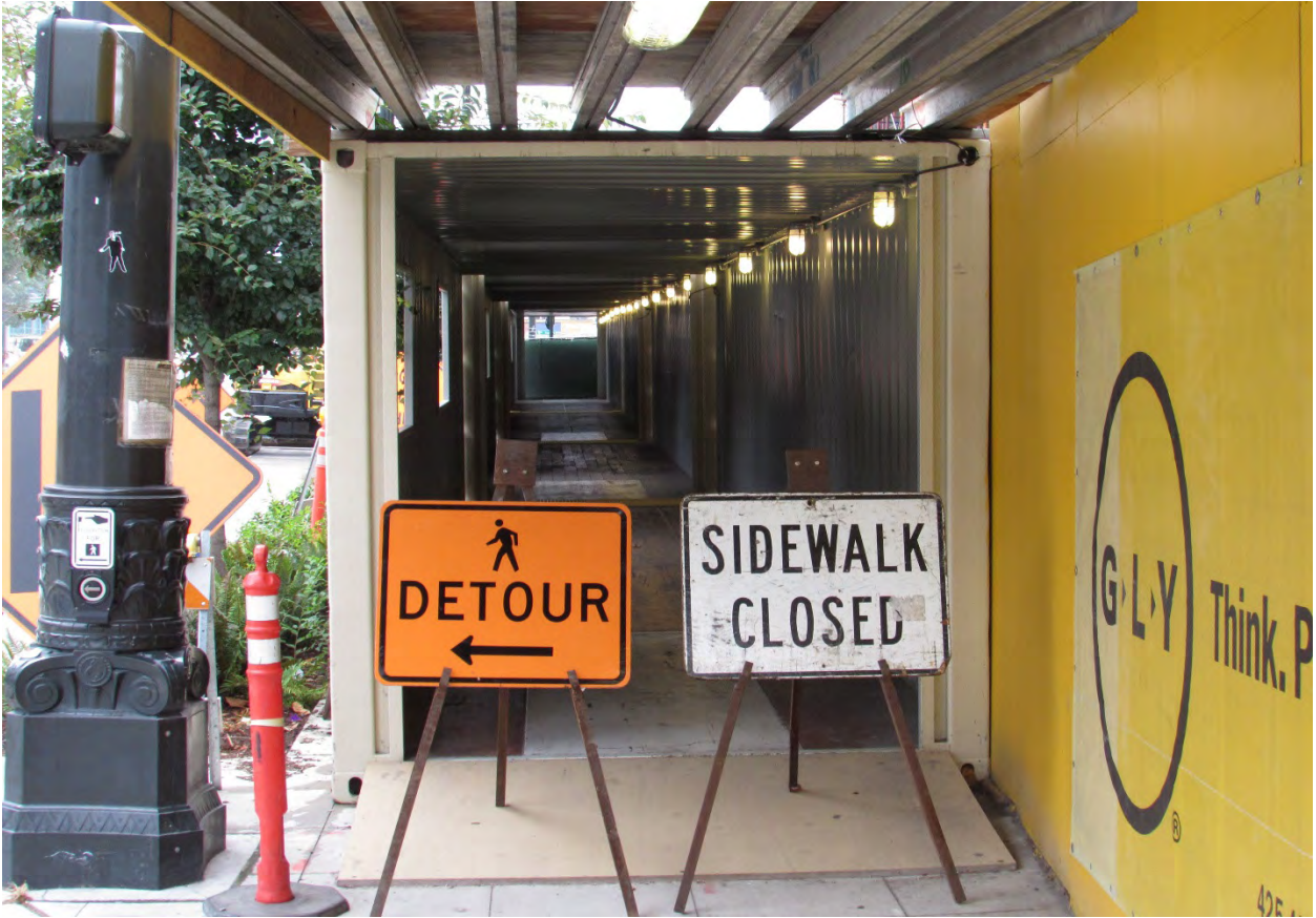
Figure 10-8: Example of Pedestrian Pathway and Falling Object Protection around construction sites (Picture Courtesy of GLY Construction)
