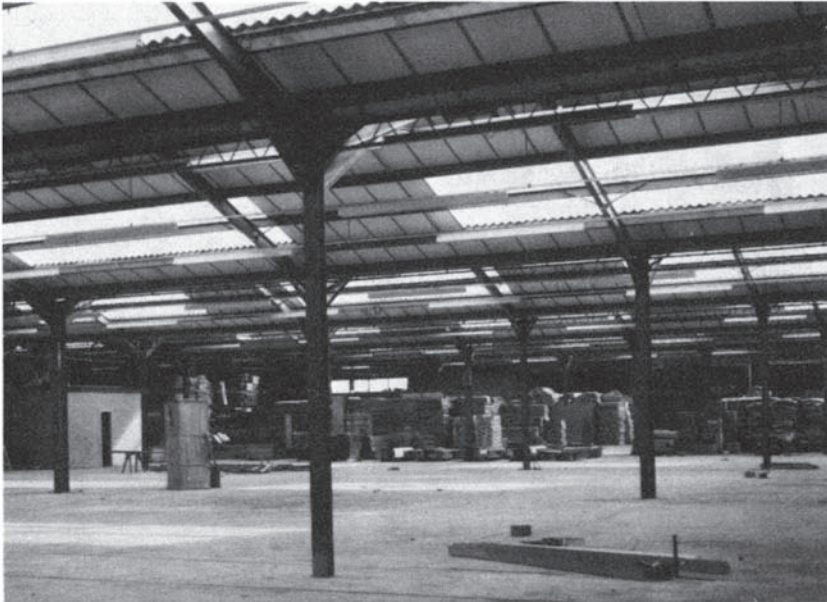
Plate 1. A typical modern factory building showing the hard reflective surfaces which promote highly reverberant conditions—concrete floor, brick walls and plastic faced plaster board roof linings
