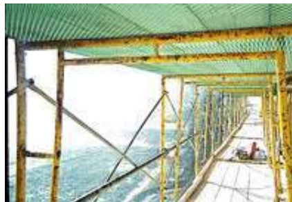
Akses di bawah perancah harus dipasang jaring dan pagar Nets and railing must be installed under the scaffolding.
