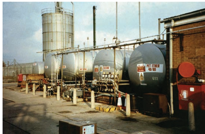
Figure 9.4 (a) Typical warehouse vehicle loading/unloading area with separate pedestrian access; (b) barriers to prevent collision with tank surrounds/bunds.
