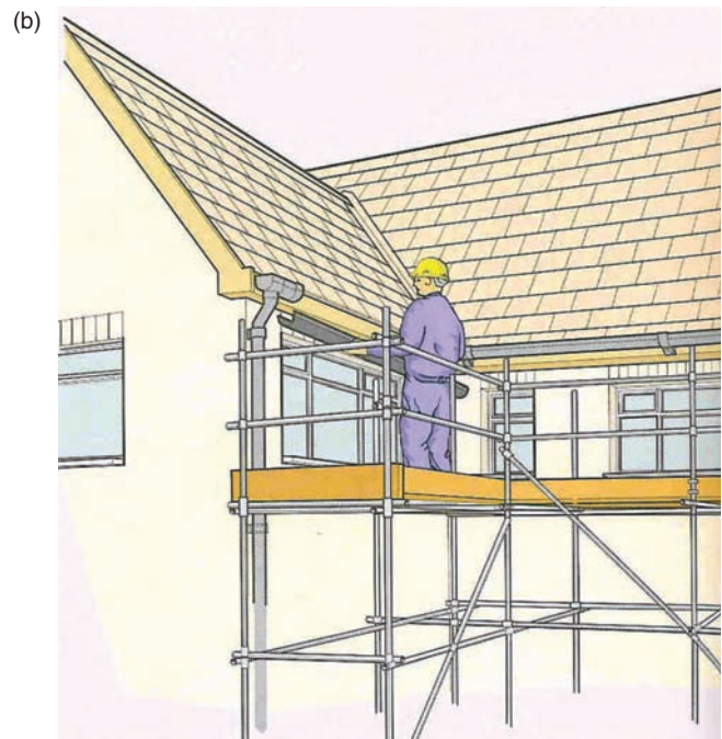
Figure 16.6 (a) Typical independent tied scaffold. (b) fixed scaffold left in place to fit the gutters.
