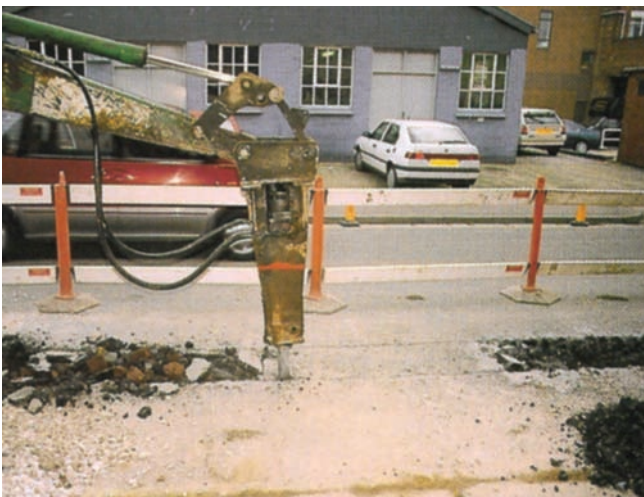
Figure 15.4 Mounted breaker to reduce vibrations.
