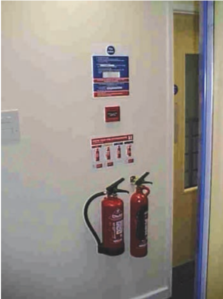
Figure 13.9 Typical fire point in offices with extinguishers, fire notice and alarm break-glass call point.
