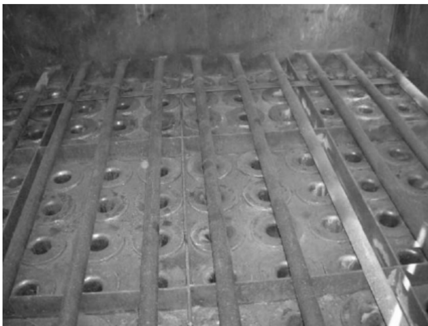
Figure 5.16. Tube sheet of dust collector, Ref. 5.25.
