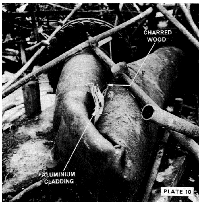
Figure 3.24. The collapsed 20 inch pipe.
