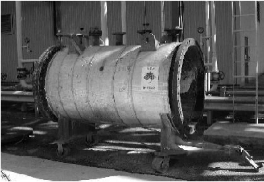
Figure 5.45. Polymer catch tank, Ref. 5.50.
