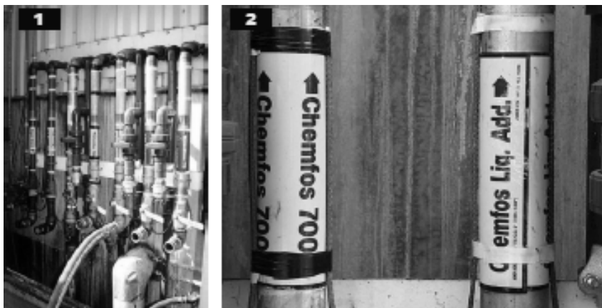
Figure 5.30. 1) Pipe connections in panel 2) Chemfos 700 and Liq. Add lines.
