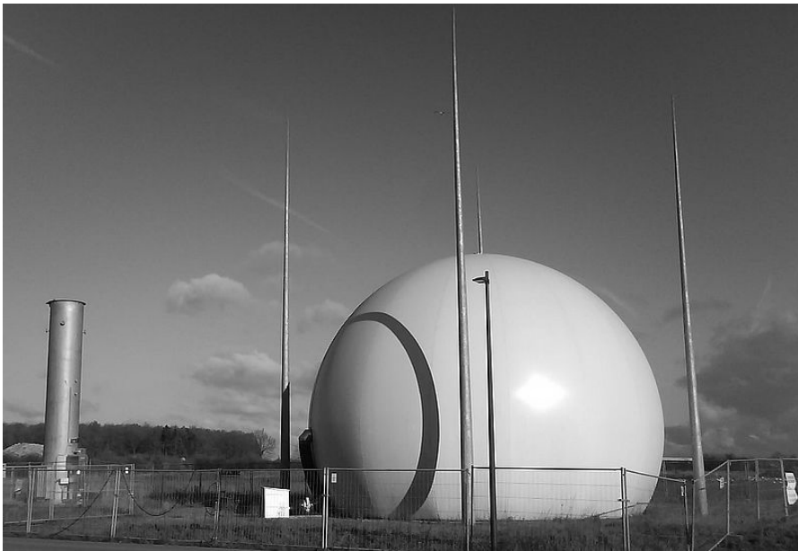
Figure 5.36 Pressurized gas storage tank.
