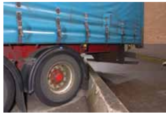
Figure 32 This concrete wheel stop helps make sure vehicles do not drive into a pedestrian area
