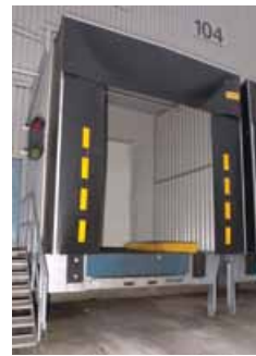
Figure 33 A well-organised loading bay, using traffic lights to inform drivers, and using visibility marking effectively
