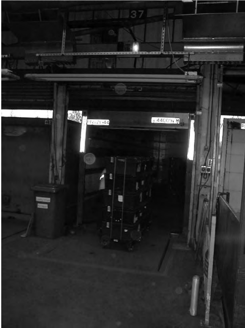
FIGURE 20.2 Dock door with RFID reader and indicator lights.
