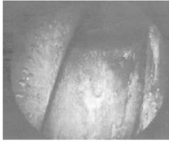
B. Erosion after 3960 hrs
