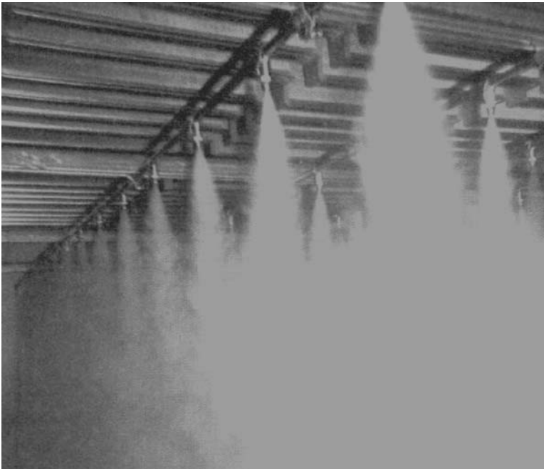
Figure 22-4. Inlet spray from evaporative cooling water nozzles.
