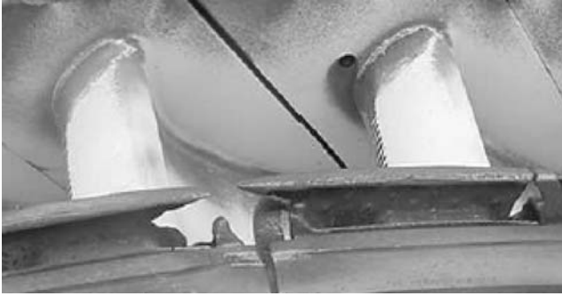
Figure 22-37. Nozzle vanes showing damage to the nozzle vane base due to high temperature.
