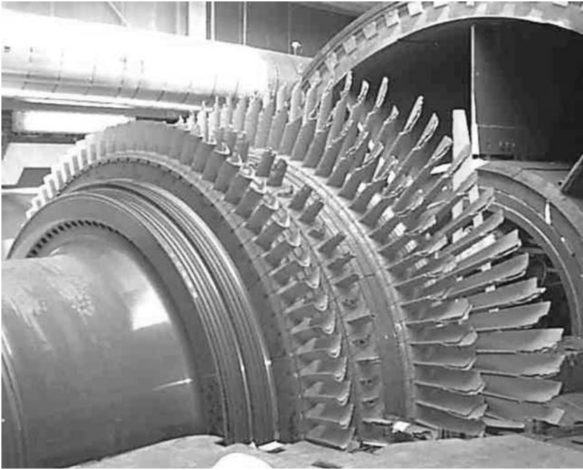
Figure 22-38. A typical gas turbine failure tip; shrouds are missing from stages two, three, and four.
