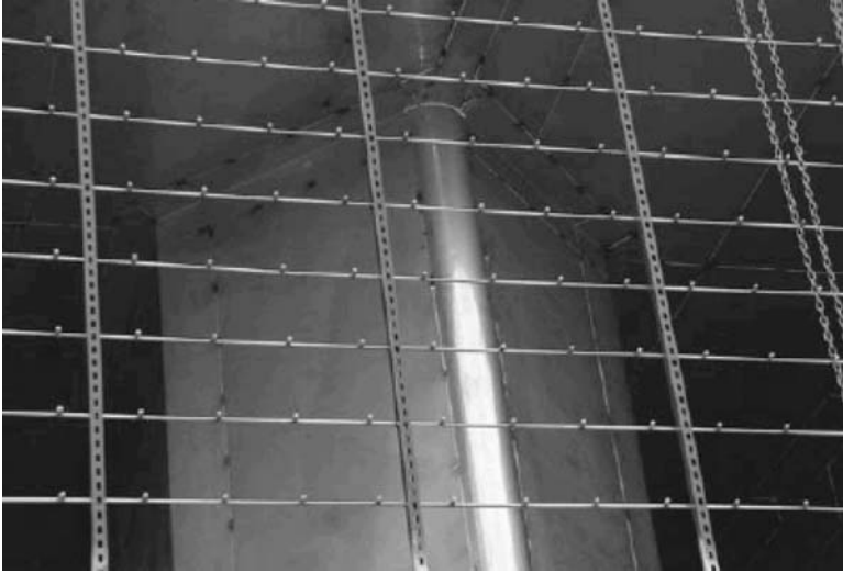
Figure 22-3. Water nozzles at the gas turbine inlet.
