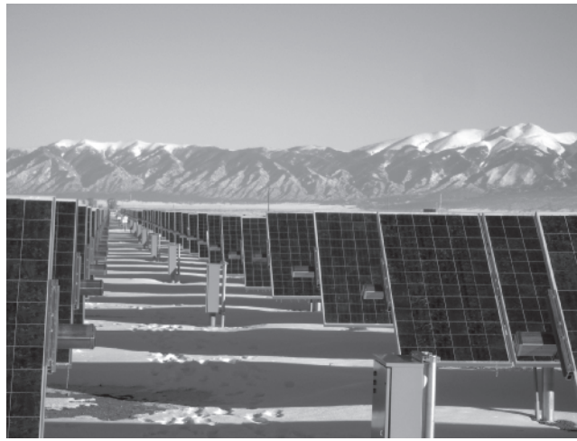
Figure 13.30 The Alamosa photovoltaic plant in Colorado.
