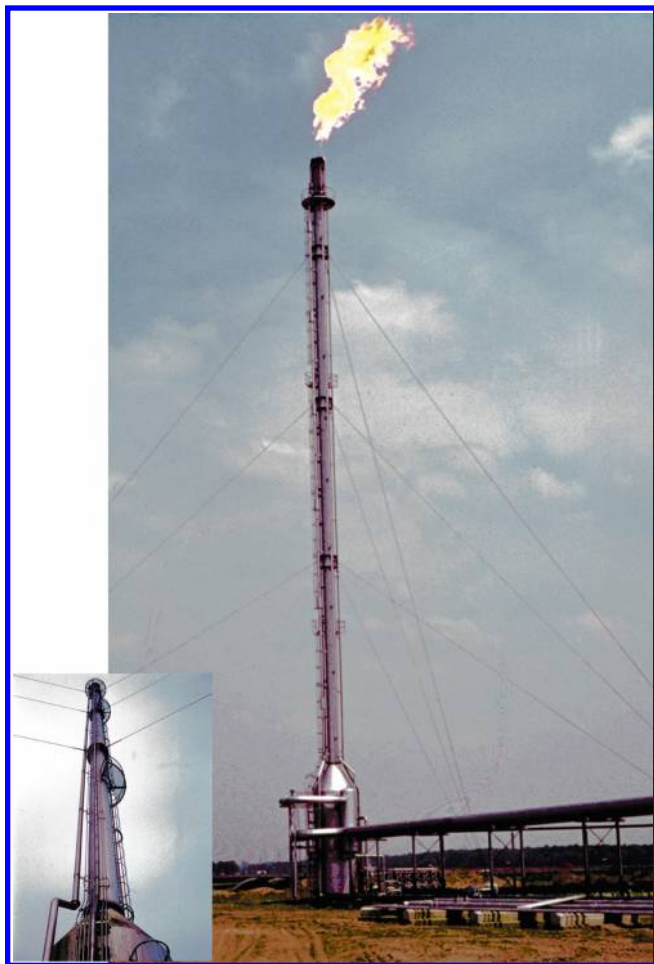
FIGURE 11.47 Guy wire-supported flare.
