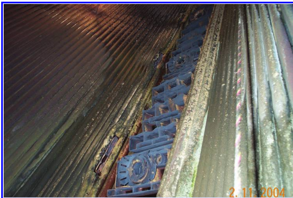
FIGURE 3.41 Corner of a T-fired boiler with tilting burners with some heat damage.
