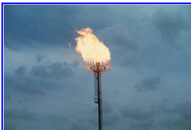
FIGURE 11.7 Elevated multipoint LRGO flare system.
