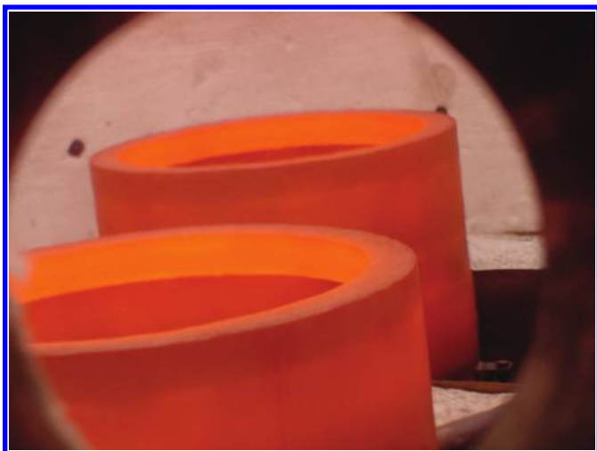
FIGURE 13.17 View inside ZULE enclosed flare.
