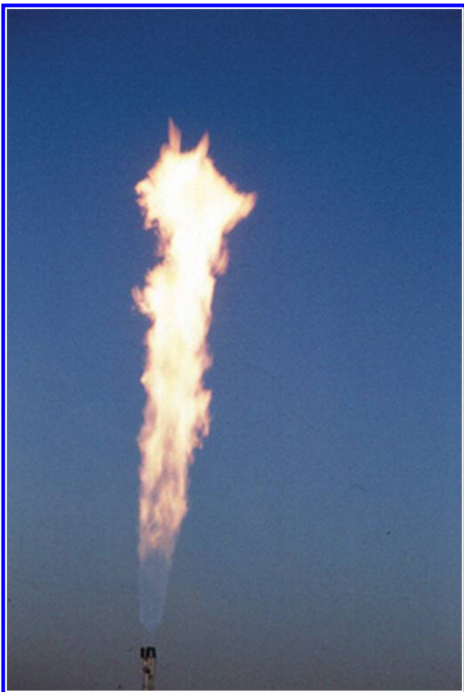
FIGURE 11.31 Hydra flare burner in an offshore location.
