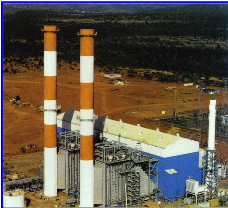
FIGURE 4.3 Combination (oil and gas)-fired duct burners at Dahbol, India. (Courtesy of Enron, Houston, TX.)
