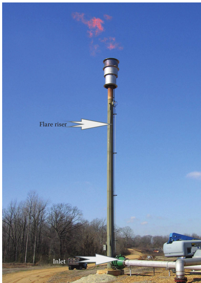
FIGURE 13.5 Elevated flare inlet and riser.
