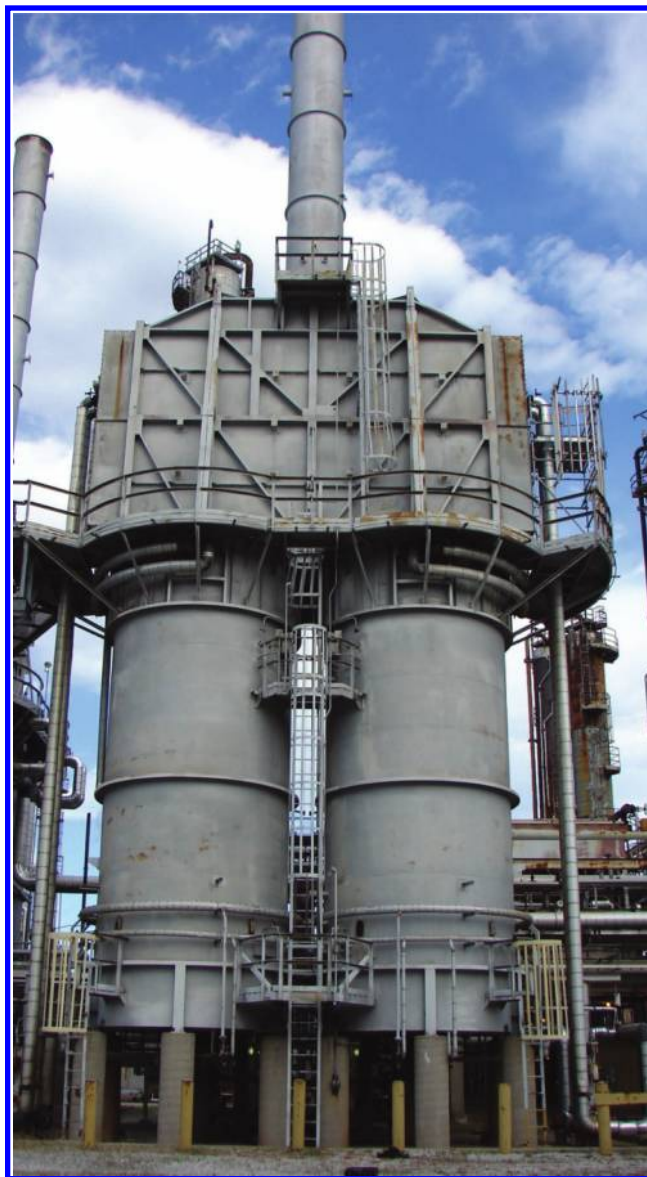
FIGURE 6.3 Two vertical cylindrical fireboxes with a common convection section.
