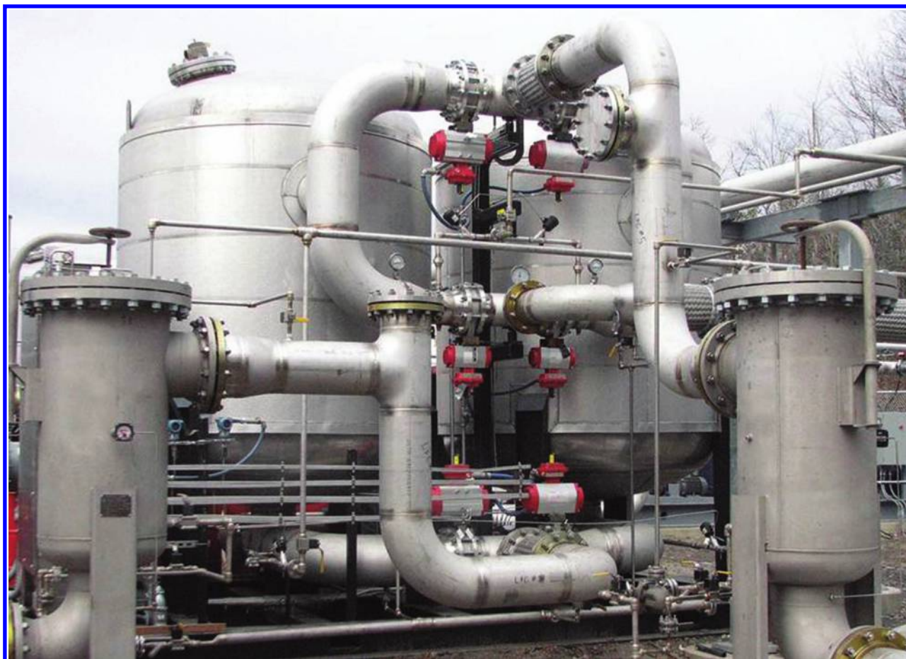
FIGURE 13.23 Siloxane removal system.
