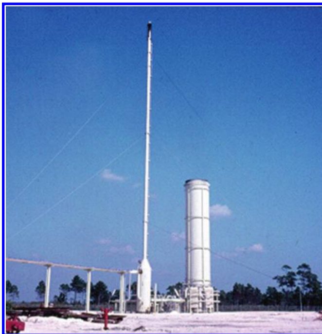
FIGURE 11.9 Combination elevated flare system (left) and ZTOF (right).
