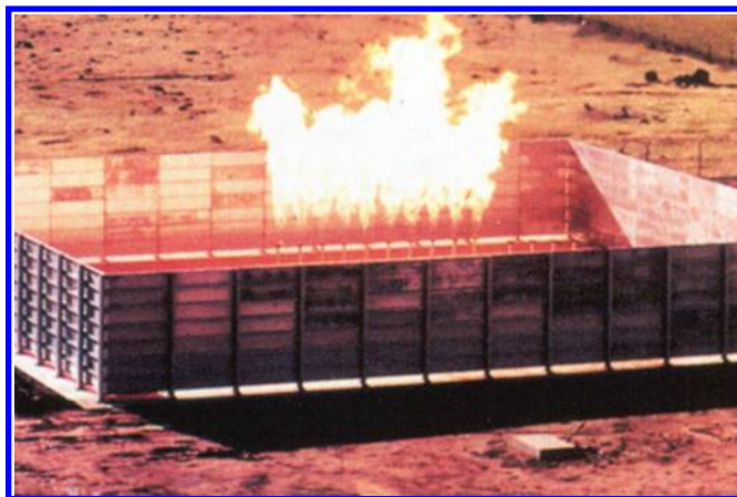
FIGURE 11.6 A grade-mounted, multipoint LRGO flare system.
