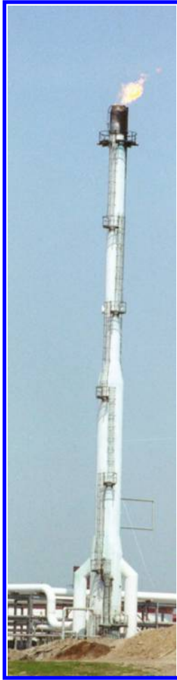
FIGURE 11.29 Air-assisted smokeless flare with two blowers in a refinery.
