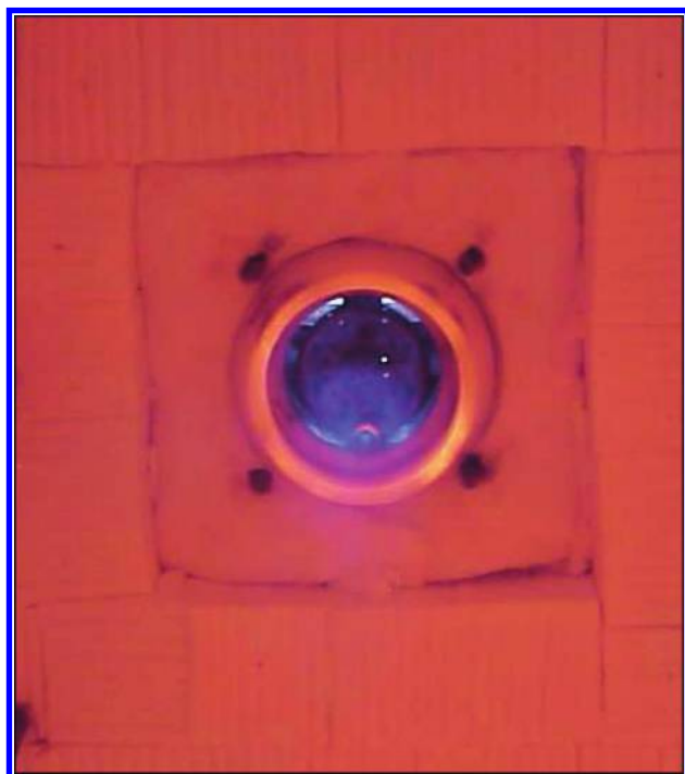
FIGURE 1.28 MDBP burner firing PSA off gas (view looking up at burner).
