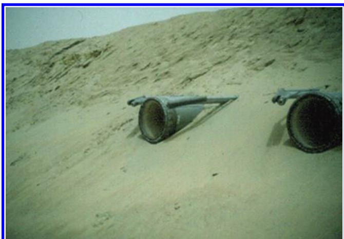
FIGURE 11.5 Typical pit flare installation.
