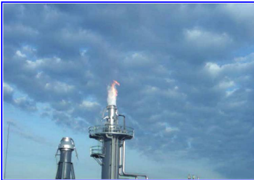
FIGURE 14.2 Example of a flare being oversteamed during testing.
