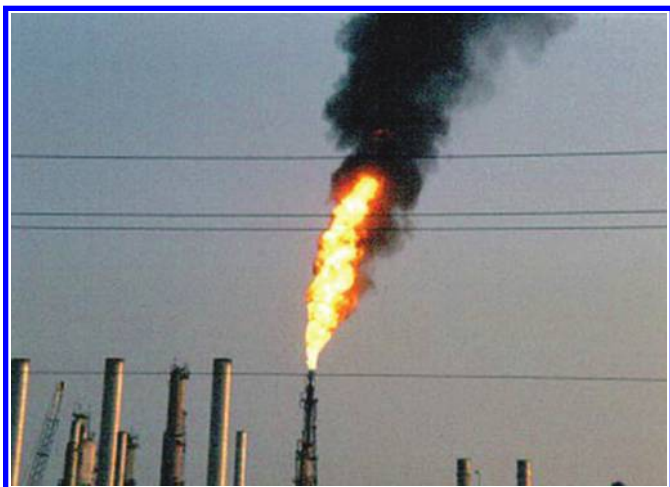
FIGURE 11.4 Typical elevated single-point flare.
