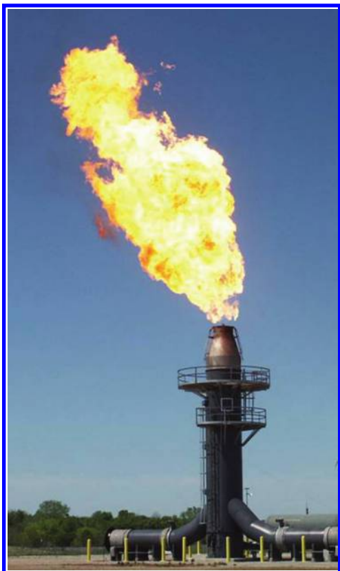
FIGURE 14.1 Example of an air-assisted flare during testing.
