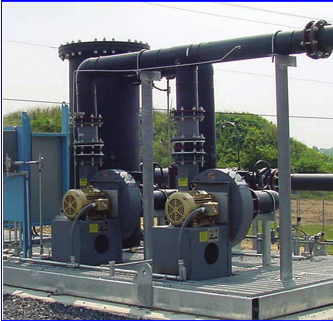
FIGURE 13.18 Single-stage fans in a landfill application.
