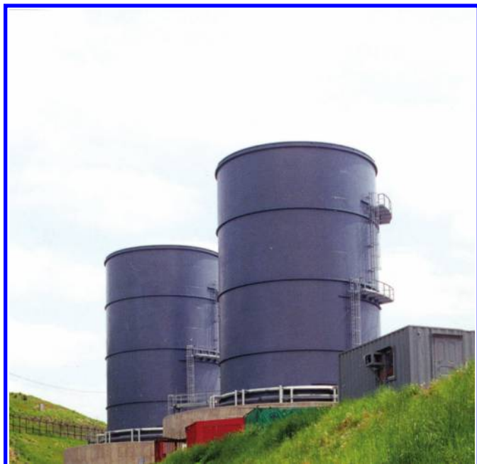
FIGURE 11.8 Multiple ZTOF installation in an ethylene plant.
