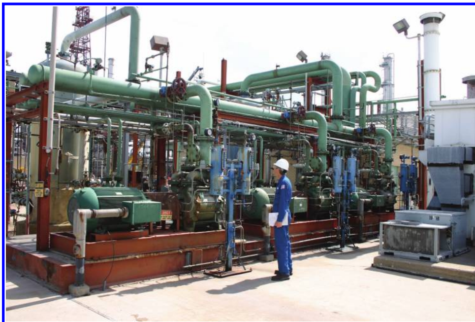
FIGURE 14.5 FGRS at FHR West Plant in Corpus Christi, Texas.
