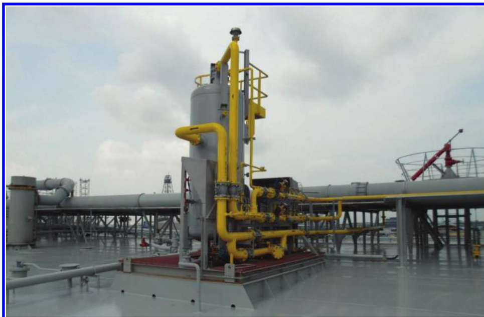
FIGURE 5.13 Hamworthy Combustion's fuel-gas knockout pot on an FSO.
