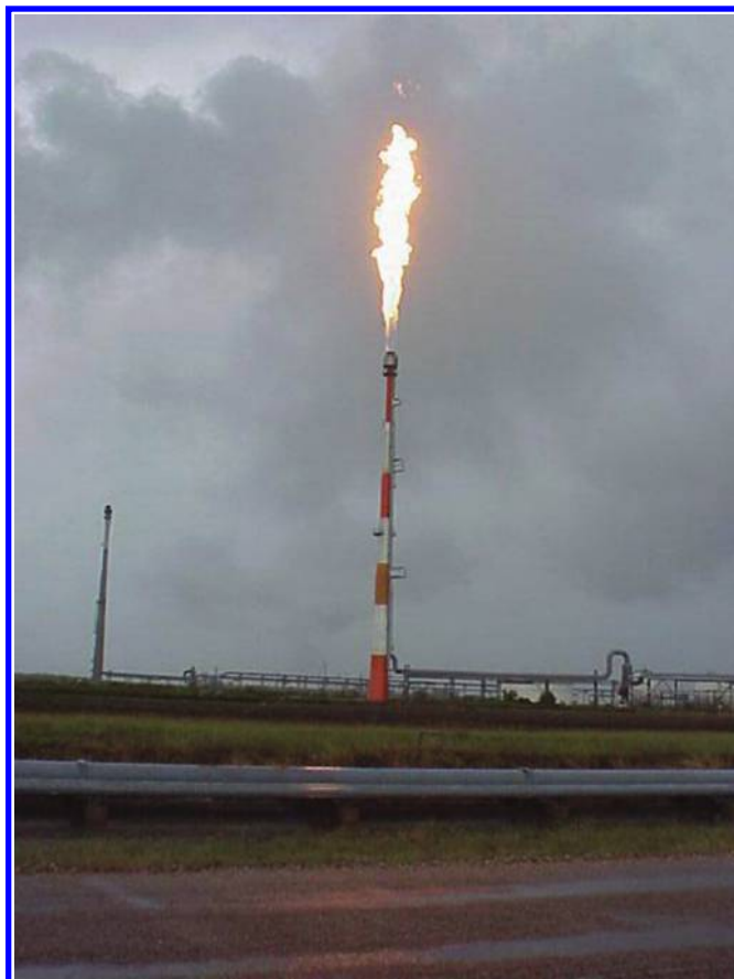
FIGURE 11.3 Major flaring event. (Note that the stack height is over 300 ft [90 m].)
