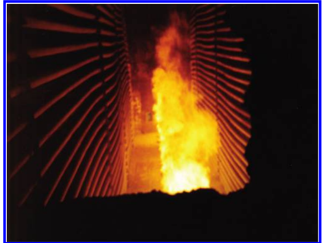
FIGURE 2.27 Flame impingement on tubes.
