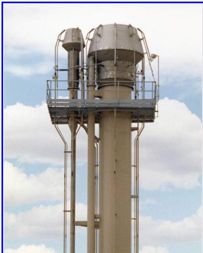
FIGURE 11.34 A RIMFIRE® endothermic flare.
