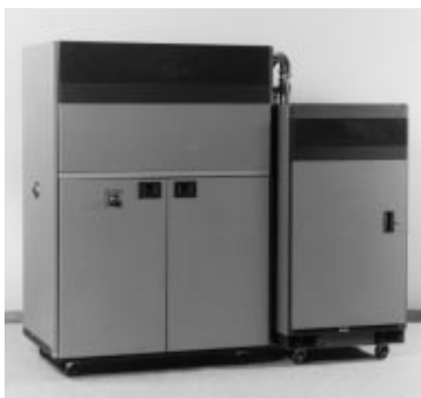
Figure 15-27: A linac RF amplifier on the left with the water pump cabinet on the right.
