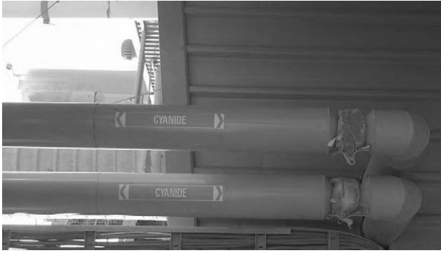
Fig. 6. Cyanide pipe colour coding and flange guards.
