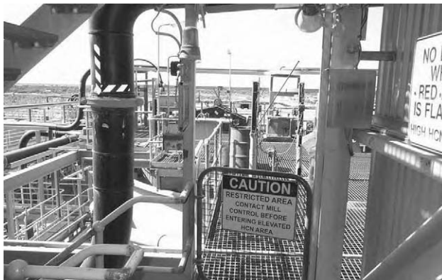
Fig. 3. Access control and warning system at entry to SDGM CIL section.
