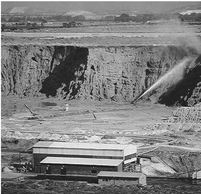
Fig. 2. Reclamation site showing remote monitor gun with main transfer station in the foreground.
