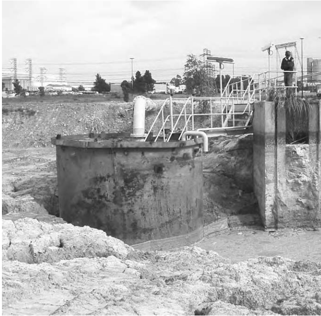
Fig. 6. Satellite pump-station (pump placed inside redundant tank which is sunk into the catchment area).
