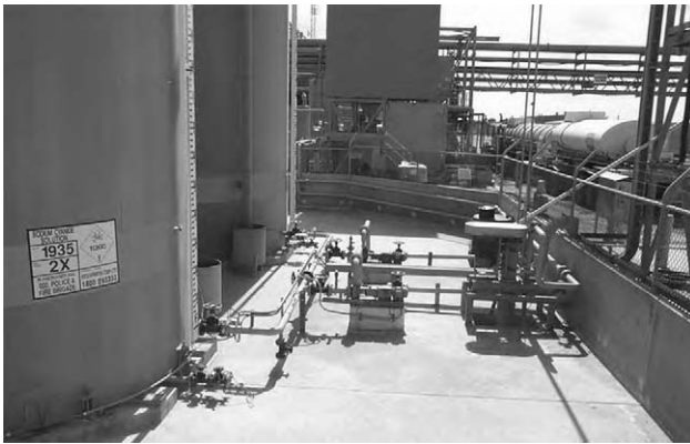
Fig. 7. Liquid cyanide storage tank and bund.
