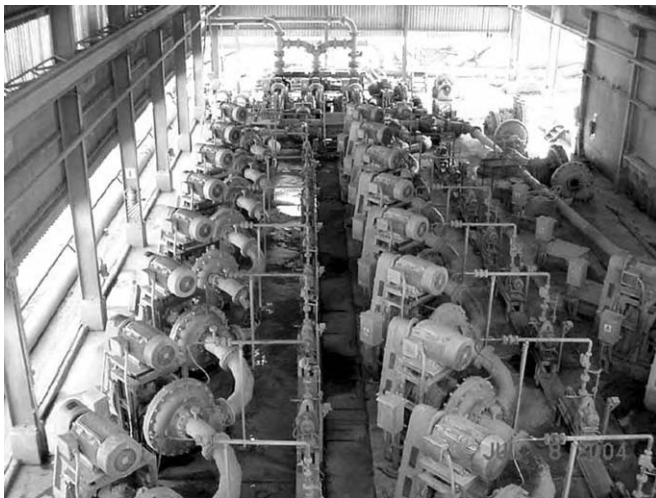
Fig. 5. Main transfer pump-station.
