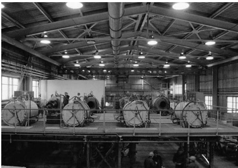
Figure 19.5 The 'Tuman' installations (The Fine Metal Powders Company's Advanced Technologies Plant).
